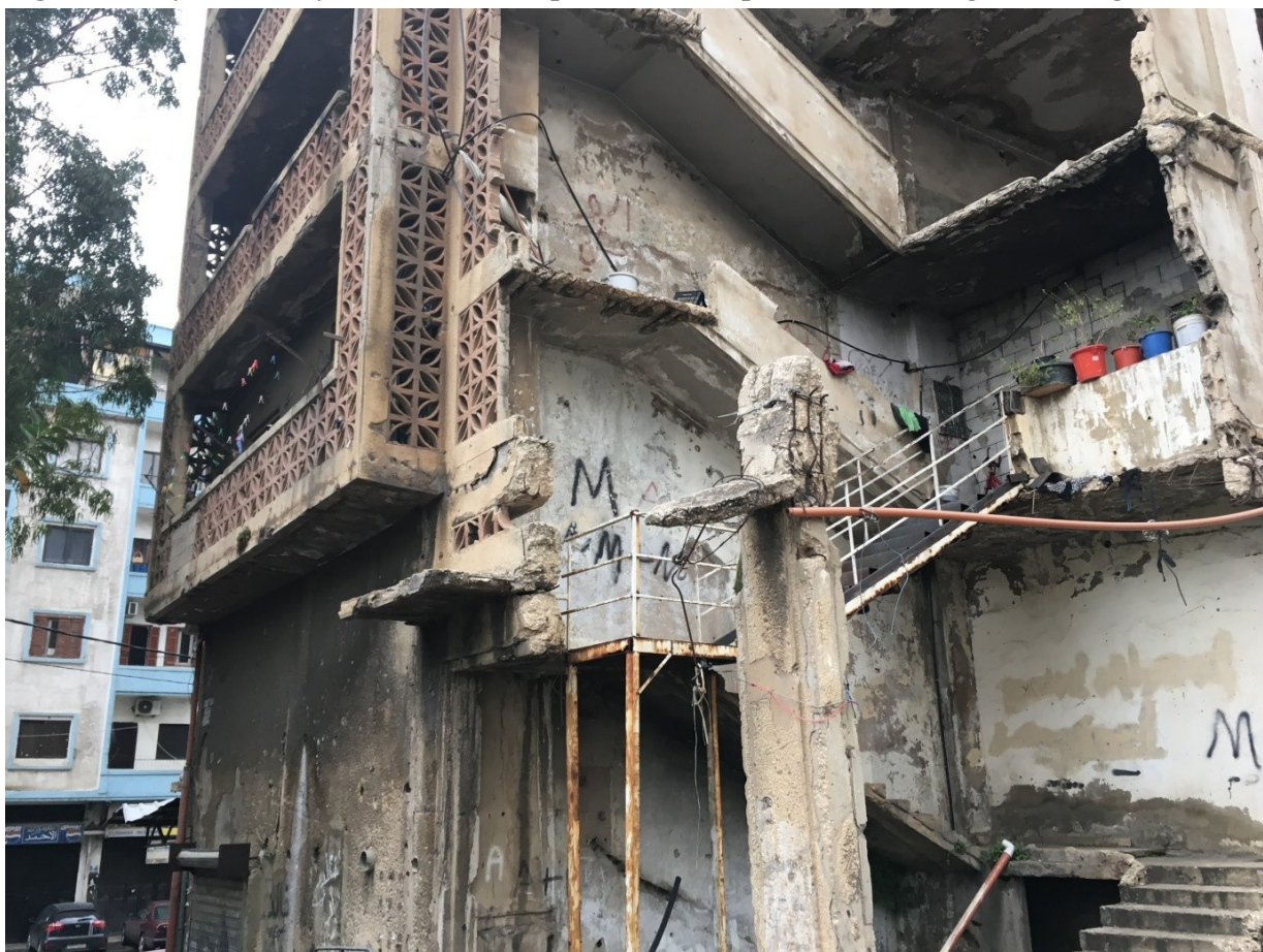
Figure 1. A Syrian family in Tebbeneh, Tripoli, rents an apartment in a fragile building structure
